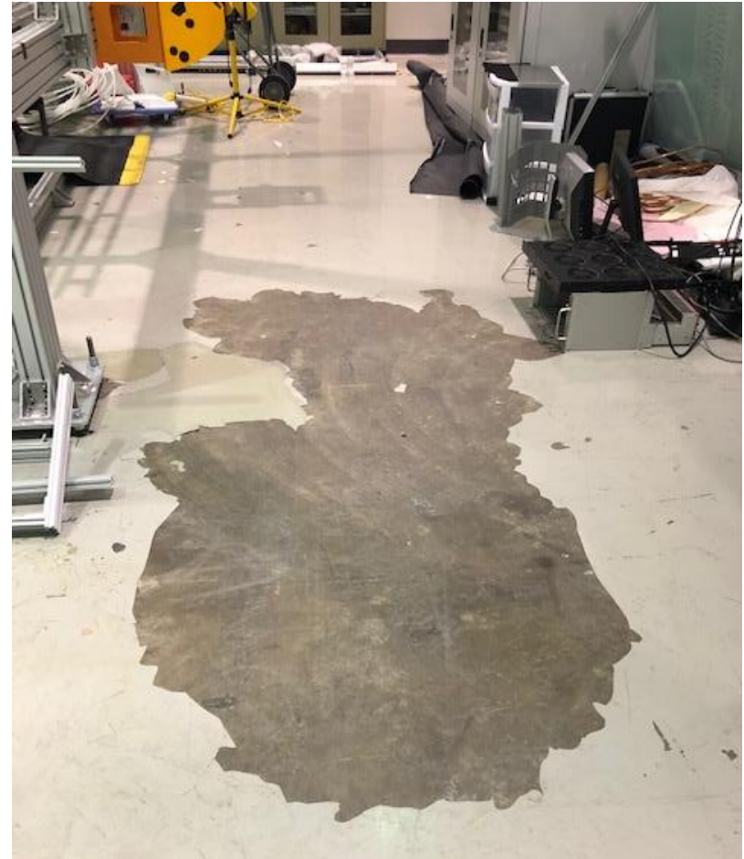
Example area where floor needs repairs in EEL 124. Area is in back of cleanroom between RICH assembly structure and aerogel dry cabinet. Area that needs repair is ~6 ft x ~3 ft.
